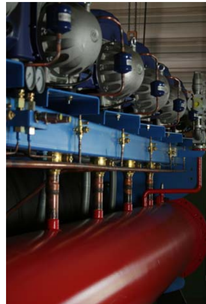
Axima 1800kW Watercooled Chiller
