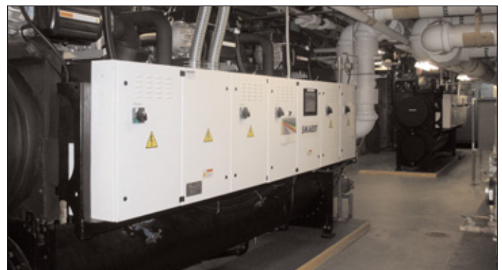
450-ton Smardt chiller featuring 5 Danfoss Turbocor compressors
