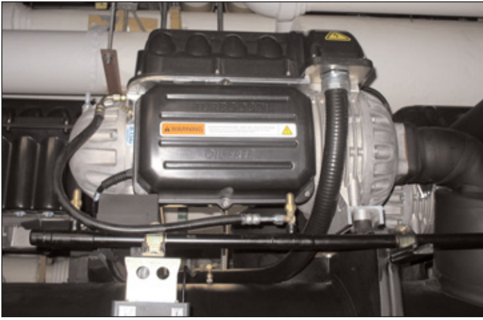
Danfoss Turboacor compressor (5 on each Smardt chiller) features oil-free compressor technology
