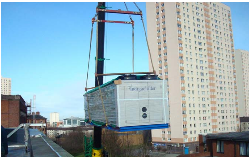
A crane lifts one of Star's Indigo chillers into position on the roof of the Curran Building of the University of Strathclyde.
